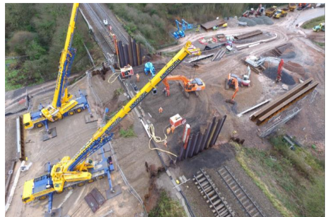
Works for the new underbridge which allows the South Bristol Link to go under the Great Western Railway
